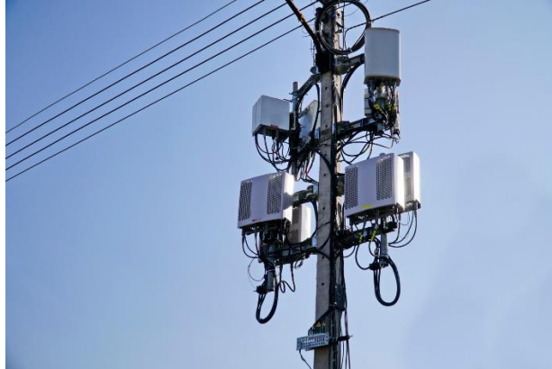
Example of improper collocation aesthetics
